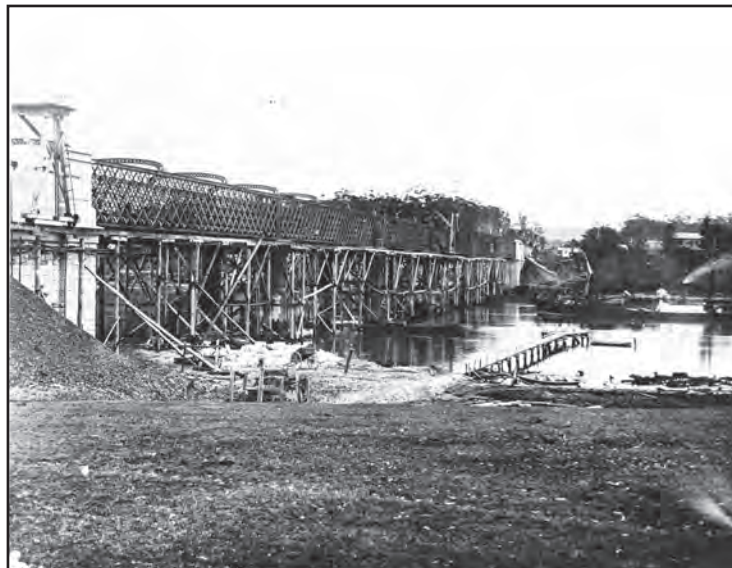
The first Meadowbank Bridge nearing completion in 1885. The timber falsework used to support the bridge components during construction is clearly evident. The view is looking north towards Meadowbank.
