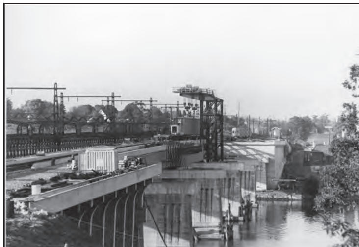
The second Meadowbank Bridge during construction in 1979. The floating crane is positioning one of the box girders onto the piers. The view is looking south towards Rhodes.
