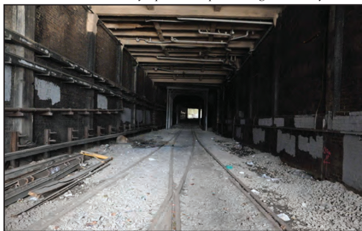
The underpass at Railway Square. The original 1855 structure is beyond the steelwork near the centre of the underpass. The double track was gauntleted following electrification of the line. Image: David Taylor
