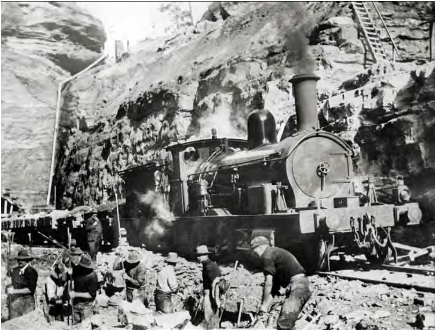
A scene during the construction of the 1913 deviation. As many as fourteen hundred men worked on the deviation, many arriving after completing the deviation around the Lithgow Zig Zag. B205 (later Z25) Class 2-6-0, 327, is seen here during the Glenbrook Tunnel construction.
