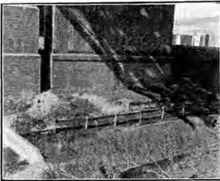
Base of one of the old Stone Arches, showing the Piers (right to left) built in 1886, 1891 and 1927.
