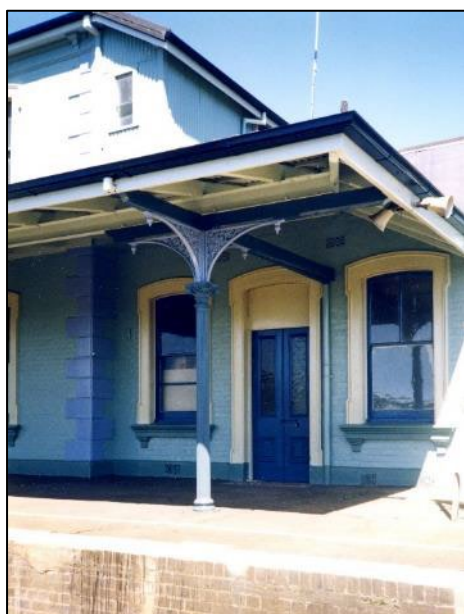
The southern end wall of the 1884 refreshment room is shown on 22 nd September 1994 and marked by the painted, sandstone quoins. The extension to the refreshment room was carried out in the 1880s as evidenced by the then prevailing design policy to indent the new extension wall where it joined the 1884 structure which was identified by the quoins. The awning over the platform was extended to cover the new pedestrian entrance to the refreshment room.
