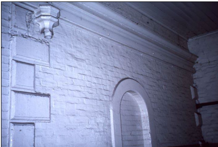
This picture shows the northern end wall of the 1880 building. The brickwork is in English bond and the building corners were emphasised by the use of sandstone quoins. Note the elegant rain head. Taken on 31 st May 2000.
