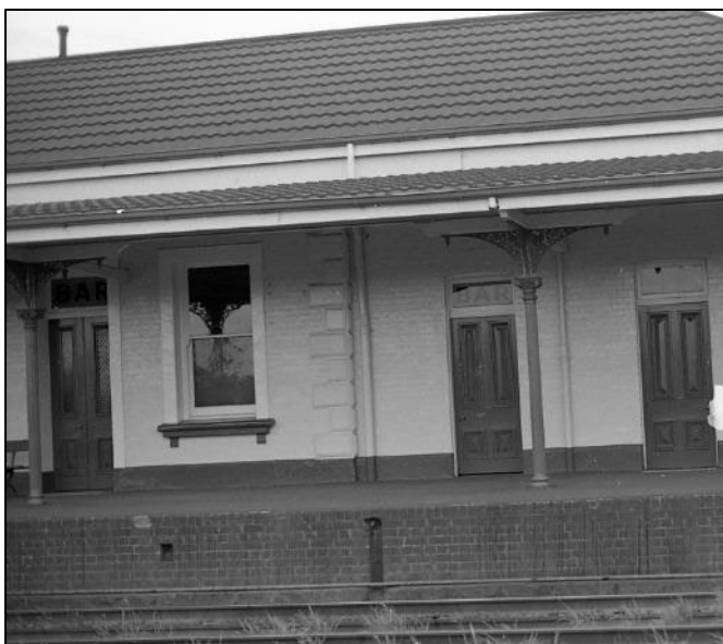
The southern end of the 1880 building is identified by sandstone quoins and the slightly recessed wall of the in-fill structure. The 1880 building was extended from that point until it met the northern wall of the 1885 built refreshment room. The roof was similarly extended. Photograph taken on 28 th May 1982.
