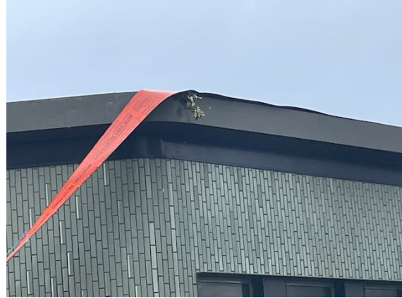
Damage to corner & tree branch in Susrey Park.
