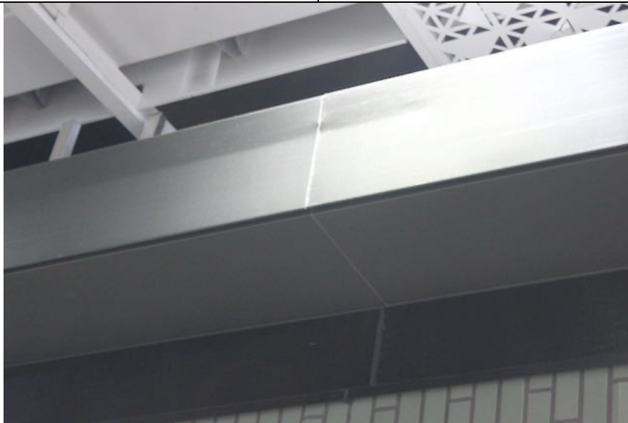
Damage to flashing on the side of the Prefab building now installed at the Down End of Union Station. 20230522
