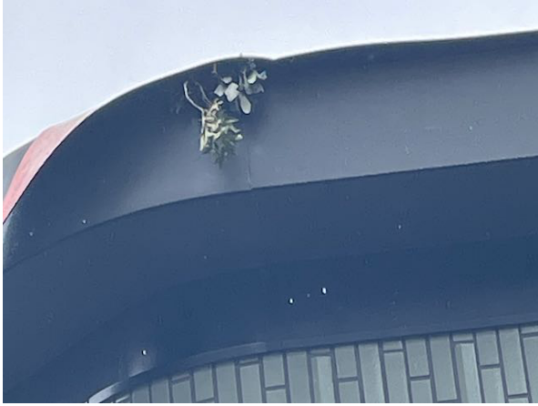
Close up of tree branch & damaged corner on PreFab Building.
