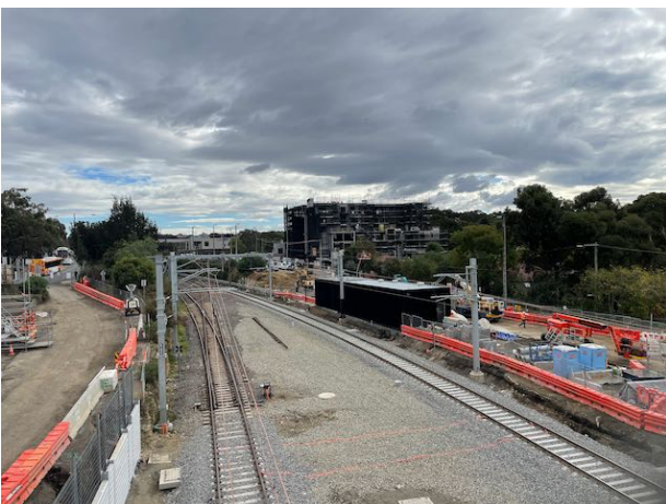
Greensborough looking in Up Direction from Concourse showing new Sub-Station on the right of track.
