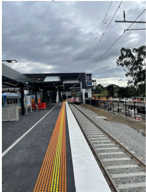
Greensborough Down Platform looking in the Up Direction showing new Concourse Building, all old Booking Office, Waiting Room & Toilets removed from Platform.
