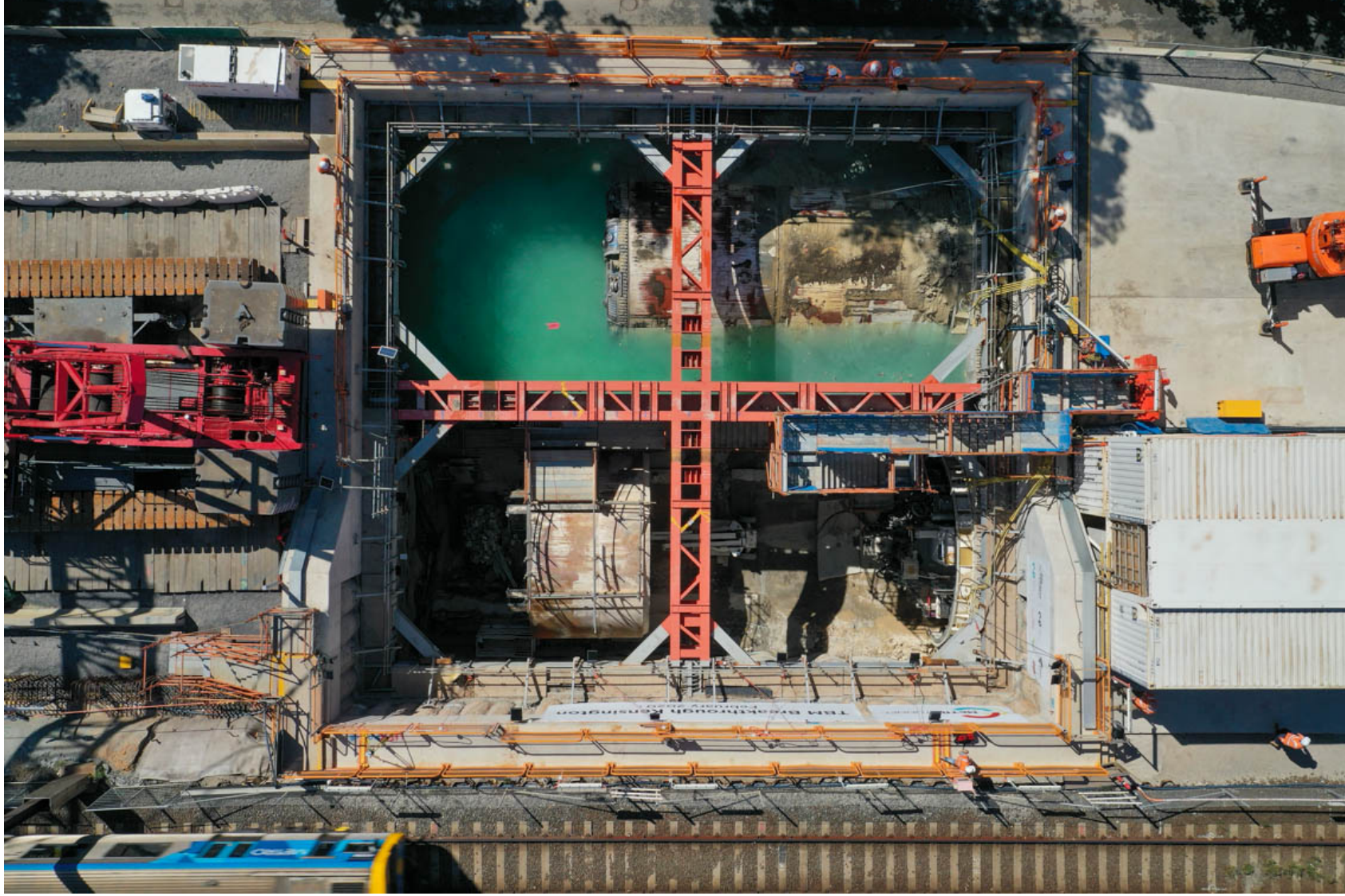
Western Portal overhead view showing Cutting Heads about to be retrieved & taken back to Arden Station site by truck for reuse on next tunnel to be bored.
