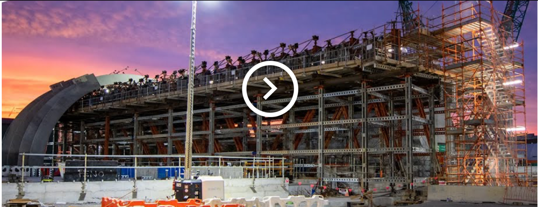
Arden Station showing framework to support the arches as they are being installed.
