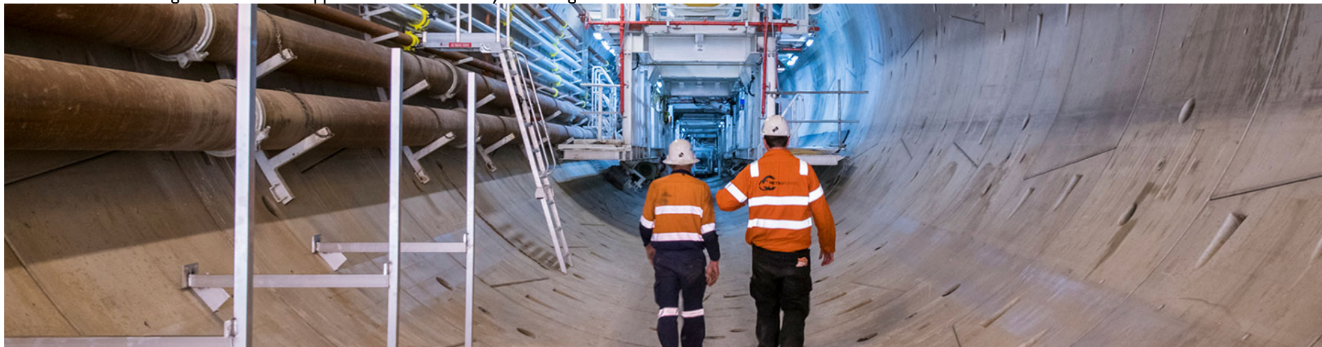
Workers in the Tunnel showing the size of Tunnel. Big build website.
