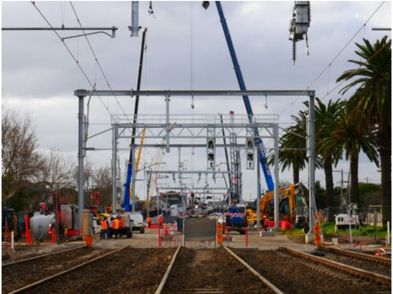
Looking in Down Direction towards Neerim Road 3 tracks going nowhere at the moment 20230711 Rod Watson Photo
