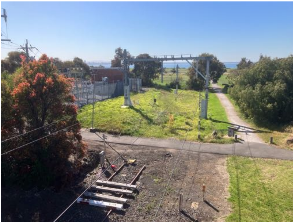
View from Footbridge at Williamstown Station down end looking towards Williamstown Pier Station JR Image
