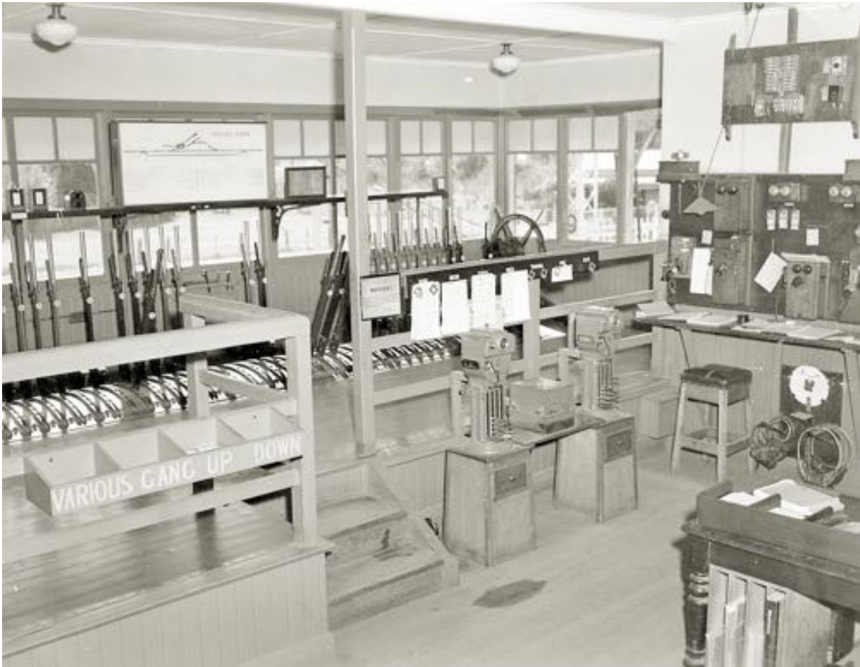
Violet Town Signal Bay c1938 Note the Signal Diagram on the wall of the Signal Bay. Image Source unknown came from Facebook?
