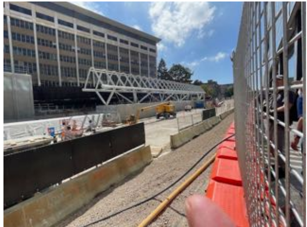
Parkville Canopy over Entrance Grattan St. GWA Image 20240131
