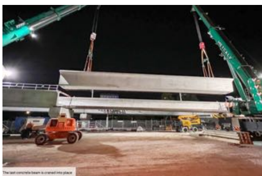
The last concrete L Beam is craned into place. Victoria's Big Build.
