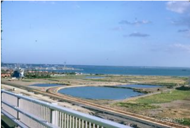
View from Westgate Bridge of Webb Dock Goods line under construction Flickr.com
