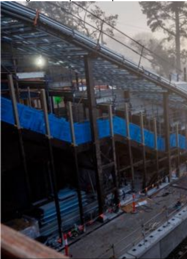
Ringwood East Looking down to Platform & Stairs 20260627 Facebook Croydon & Ringwood Level Crossing Removal Updates Group
