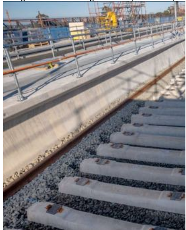
Croydon on the Platform showing Sleepers laid waiting for rail 20260627 Facebook Croydon & Ringwood Level Crossing Removal Updates Group
