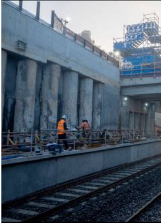
Ringwood East on the Platform under the Concourse 20260627 Facebook Croydon & Ringwood Level Crossing Removal Updates Group
