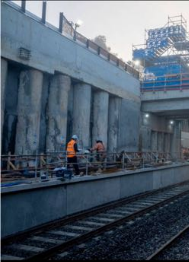
Ringwood East on the Platform under the Concourse 20260627 Facebook Croydon & Ringwood Level Crossing Removal Updates Group
