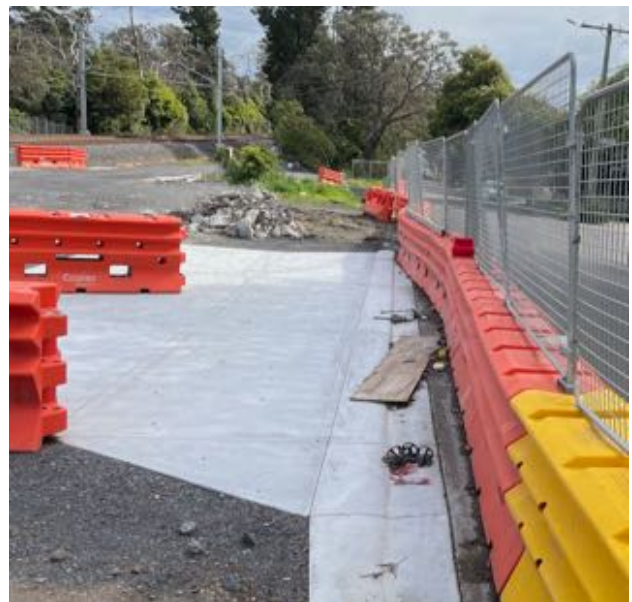
Road Rail Access Pad RWEI Ringwood East showing Driveway in from Patterson St Ringwood East. GWA Photo
