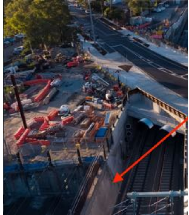
Bedford Road Rail Underpass looking South in Down Direction showing Siding Wall built c1980 against Down Track Bigbuild Victoria
