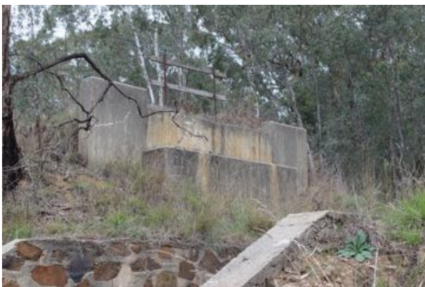
Bridge footings of 5'3" Railway Bridge by the side of the Goulburn Valley Highway. GWa pic 20140419
