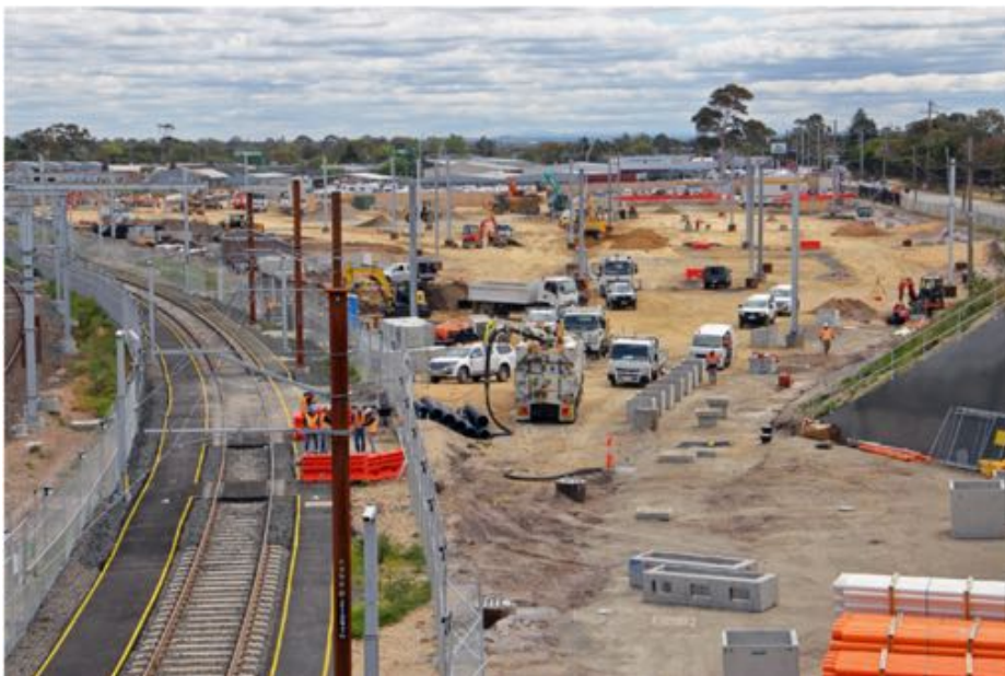
Construction works for the new stabling sidings at Kananook. Thursday 14 th November 2019 Ian Green Photo vicsig.net
