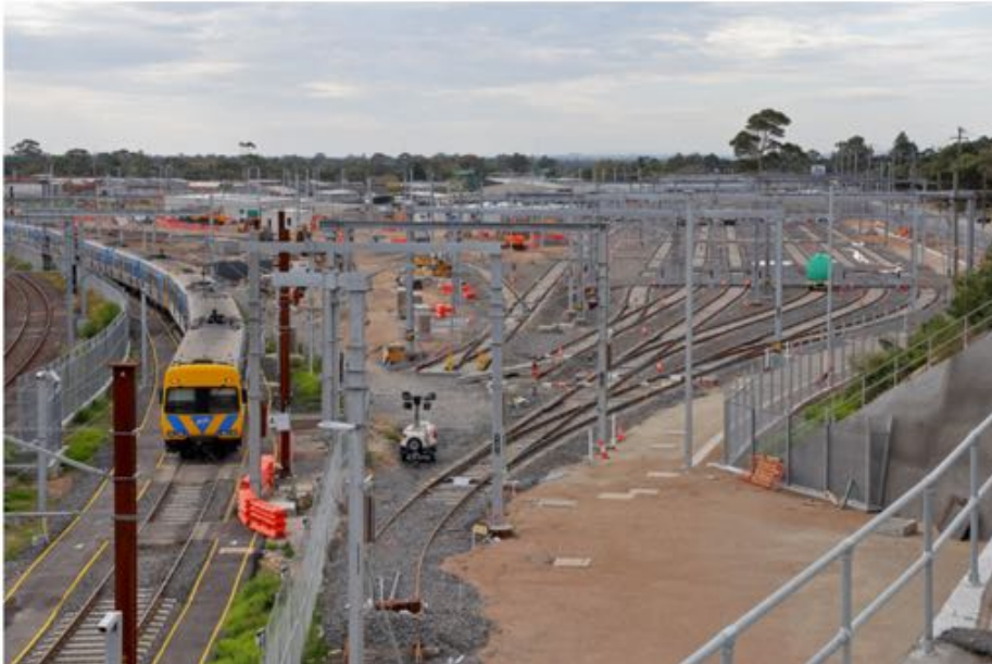
New Stabling Sidings under construction at Kananook Tuesday 14 th April 2020 Ian Green Photo vicsig.net
