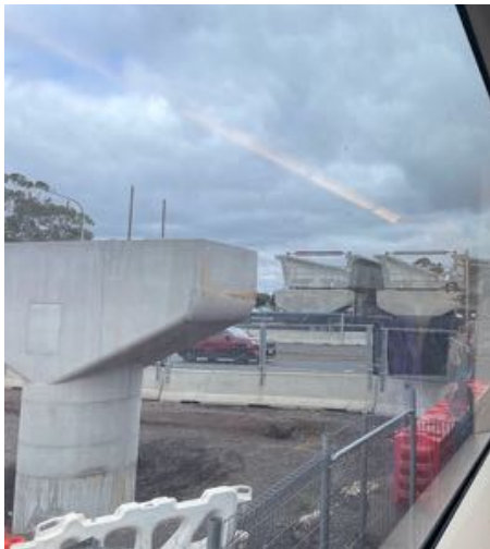
Elevated rail 4 GWa Pic 20251222
