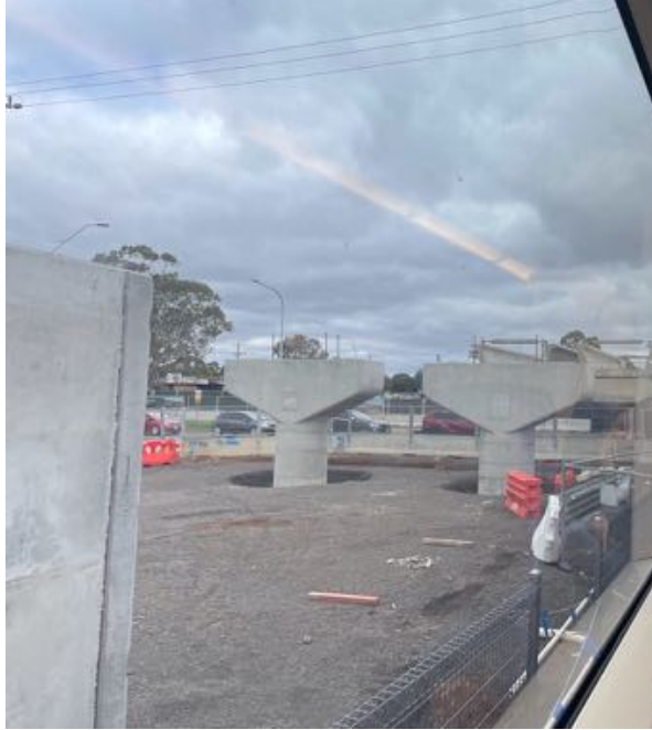
Elevated rail 2 GWa Pic 20251222
