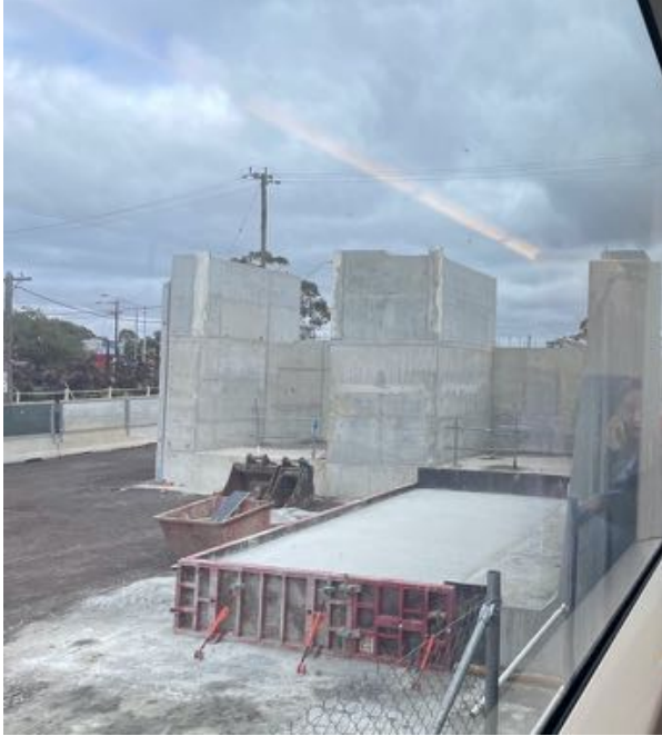
Elevated rail 1 GWa Pic 20251222
