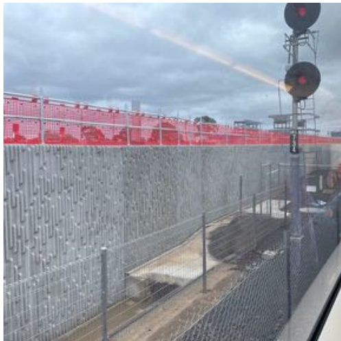
Elevated rail 5 GWa Pic 20251222
