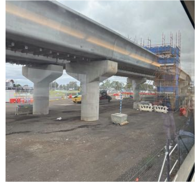
Elevated rail 3 GWa Pic 20251222
